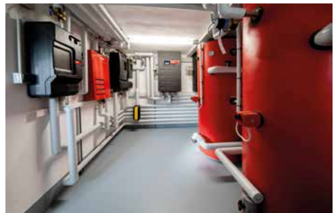
Where oil tanks once stood, there is now a completely new system consisting of heat pump cascades, TransTherm® modules and water tanks.
