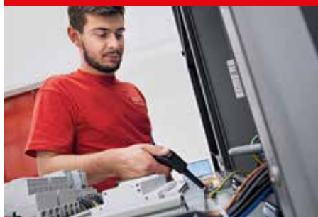
Electrical assembly | Insulation measurement
